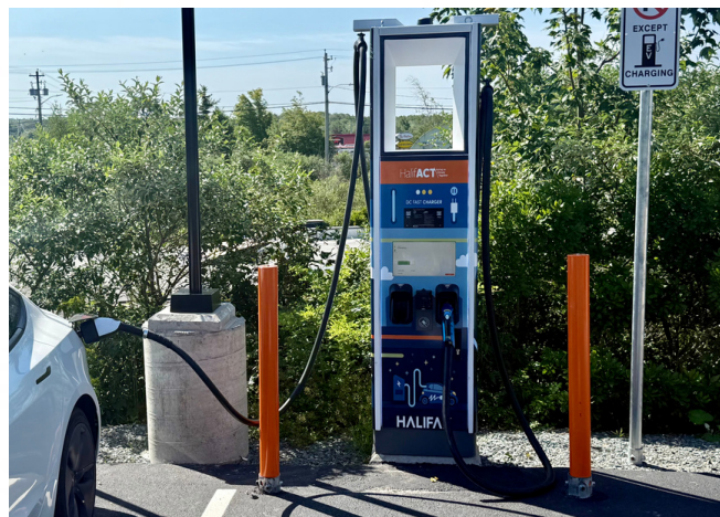
Highmark Power, HRM Fast Charger, Upper Tantallon
