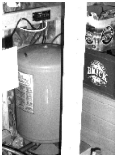
Clockwise from top: PV/battery controller, water tank, water pump pressure switch, battery box, and beer.
